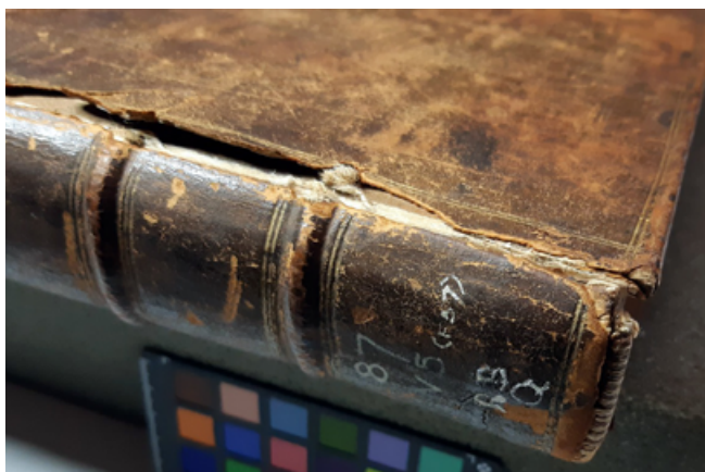
Figure 2: Before treatment. Loss of leather at the front joint and at the tail cap, but the endband was still intact. Image courtesy of Book Conservation Services.
